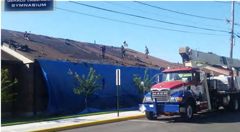
(PHOTOS, TOP) Work is currently underway this summer to transform the gym at Wood-Ridge Jr./Sr. High School into a state-of-the-art facility for students, teams and spectators; work at Catherine E. Doyle School (3RD PHOTO) includes a new boiler and new roof.
